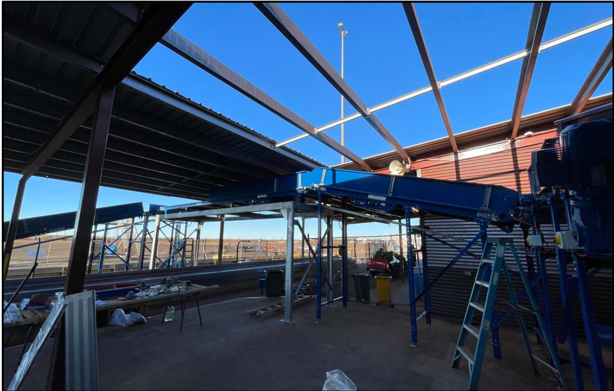
Baggage Carousel – Removal of the existing roof to heighten and extend towards the Apron
