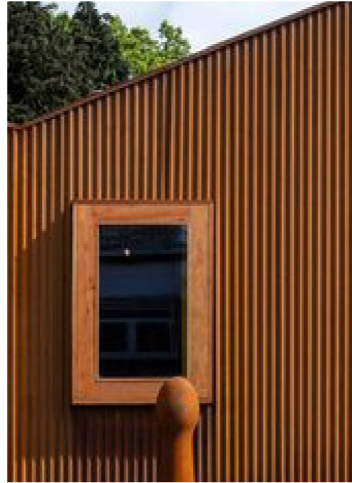
Rusted corrugated steel sheets
